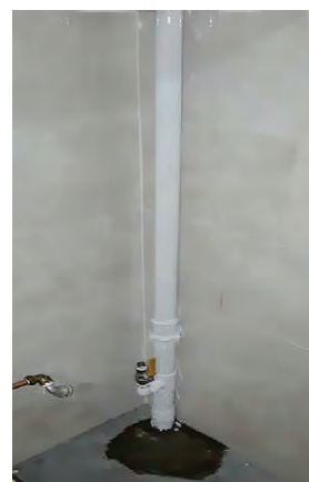
Example of gas riser pipe in kitchen of HDB flat
